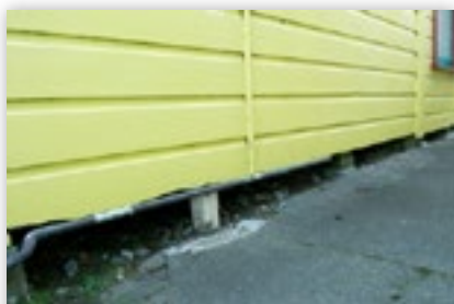
Figure 7: Areas of subfloor space with insufficient clearance
