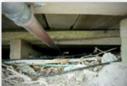
Figure 8: Areas of subfloor space with insufficient clearance
