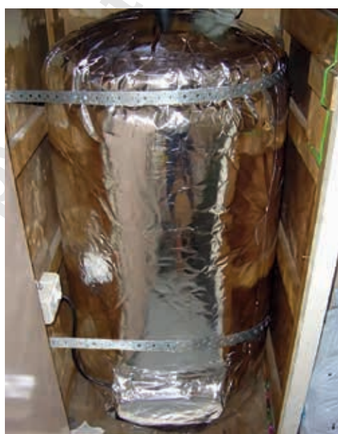
Figure 35 – Insulated hot water cylinder
